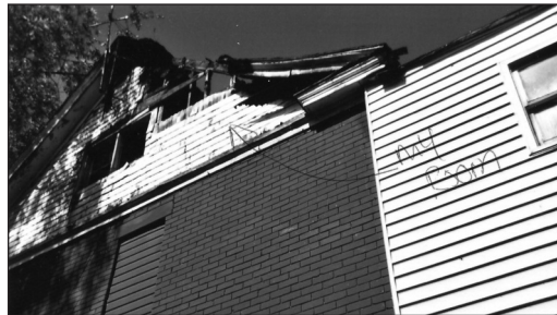
Flames spread quickly from the first floor of this 2.5-story house to its attic, where a woman was sleeping.
